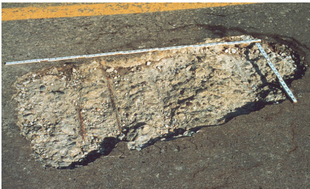
Figure 133. Typical deck spall with exposed rebar. Locations 3 and 4.
