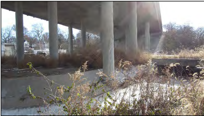
Figure 169. Cracking in RC column at Bent 7 for Bridge Number 15558X.
