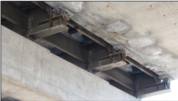
Figure 174. Typical pot bearings with surface rust for Bridge Number 15558X.
