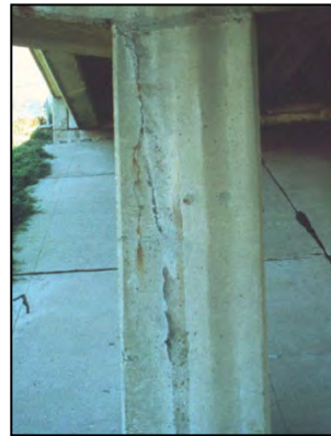
Figure 139. Crack in Pier 3 column. Location 3.
