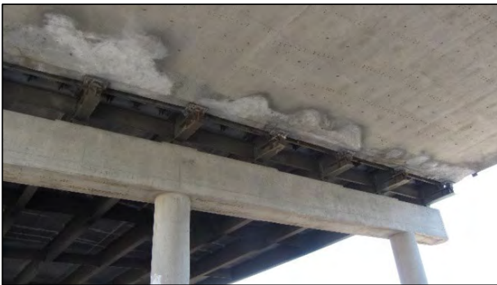
Figure 167. Unsound patched areas and efflorescence on underside of RC voided slab for Bridge Number 15558X.
