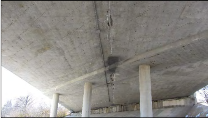
Figure 166. Spalls with exposed rebar on underside of RC voided slab for Bridge Number 15558X.
