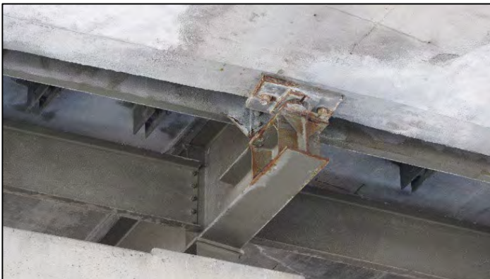
Figure 165. Surface corrosion on cantilever steel beam ends for Bridge Number 15558X.
