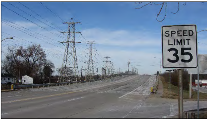
Figure 183. Approach roadway with speed limit sign for Bridge Number 15558X, looking north.
