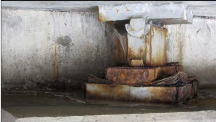
Figure 173. Typical rocker bearing with movement restricted by pack rust for Bridge Number 15558X.
