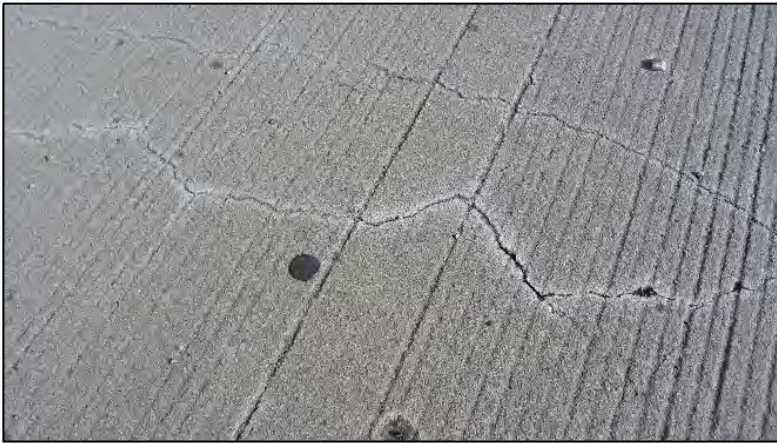
Figure 163. Closer view of cracking in wearing surface for Bridge Number 15558X.
