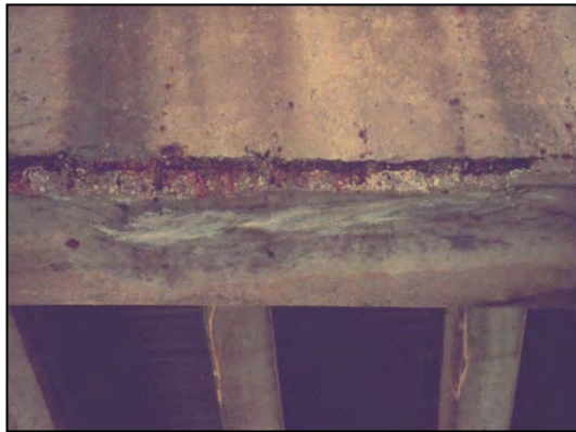
Figure 138. Spall in Pier 2 cap beam. Location 1.
