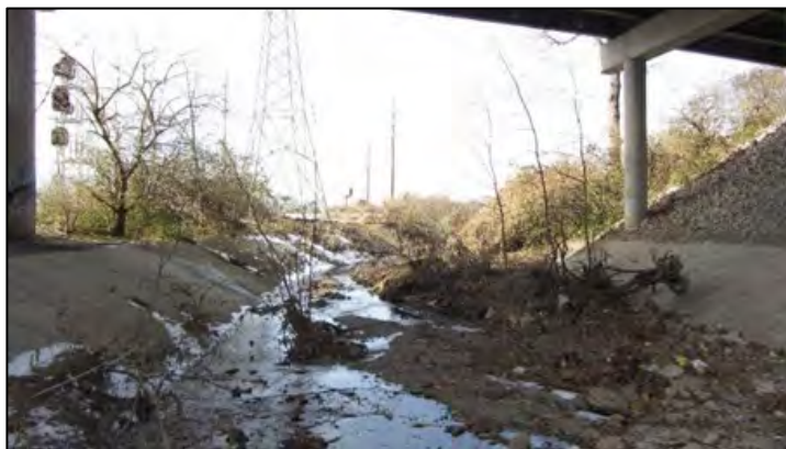
Figure 178. RC lined channel with debris and vegetation for Bridge Number 15558X.
