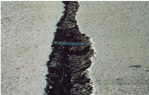
Figure 132. Deck spalling along joint. Location 2.
