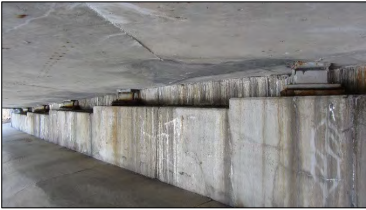
Figure 168. Cracking in south RC abutment for Bridge Number 15558X.
