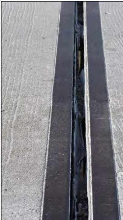
Figure 177. Strip seal ripped and punctured completely through for Bridge Number 15558X.
