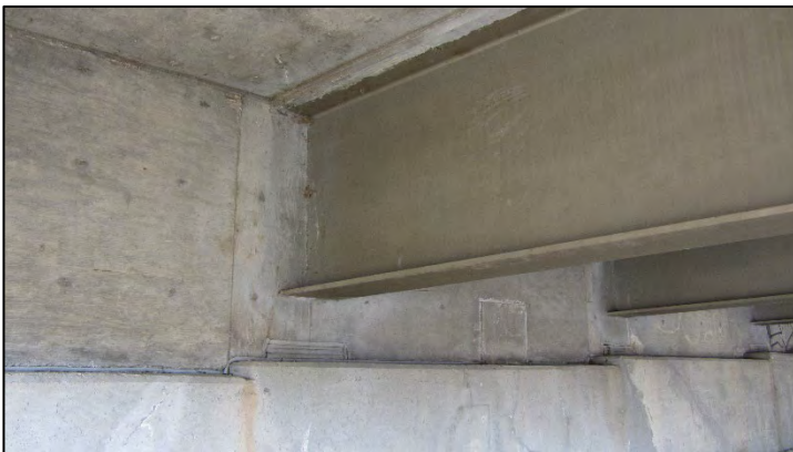
Figure 170. Cracking in north RC abutment for Bridge Number 15558X.
