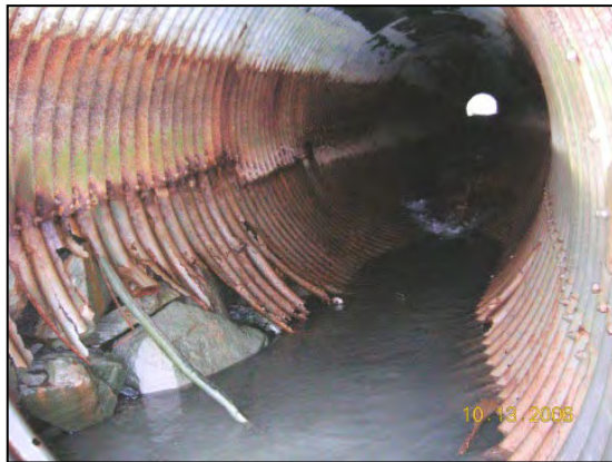
Figure 141. Corroded pipe culvert invert. Location 1 and 3. (Source: Alaska DOT)
