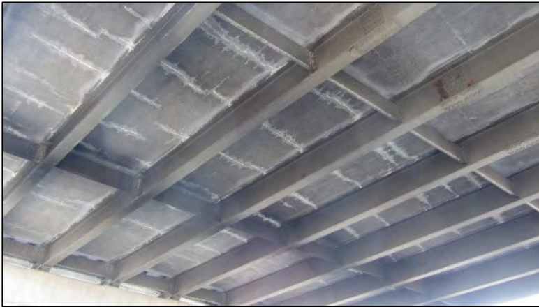
Figure 161. Transverse cracking with efflorescence on underside of RC deck for Bridge Number 15558X.
