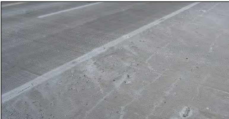
Figure 162. Longitudinal cracking in wearing surface for Bridge Number 15558X.
