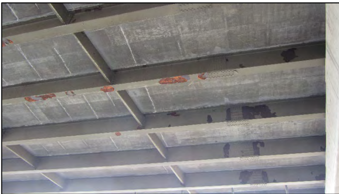
Figure 164. Spot surface corrosion on steel beams for Bridge Number 15558X.
