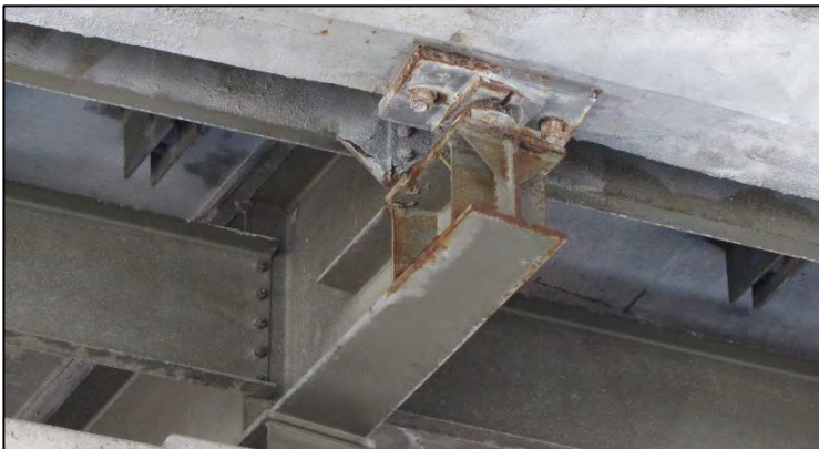
Figure 175. Closer view of typical pot bearings with surface rust for Bridge Number 15558X.
