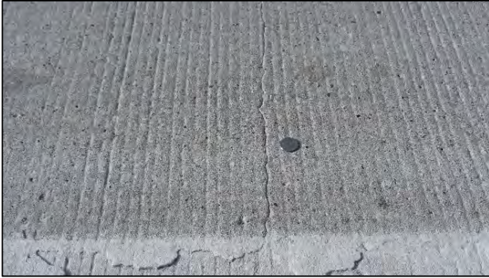
Figure 160. Transverse cracking in top of RC deck for Bridge Number 15558X.
